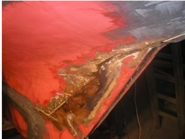
Exposed Rotten Horn Timber and Deadwood From Below
